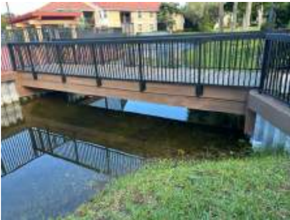
Pedestrian bridge at pond is in good conditions. Reserves includes redecking and railing replacement. Also includes structure repairs/replacement when needed.
