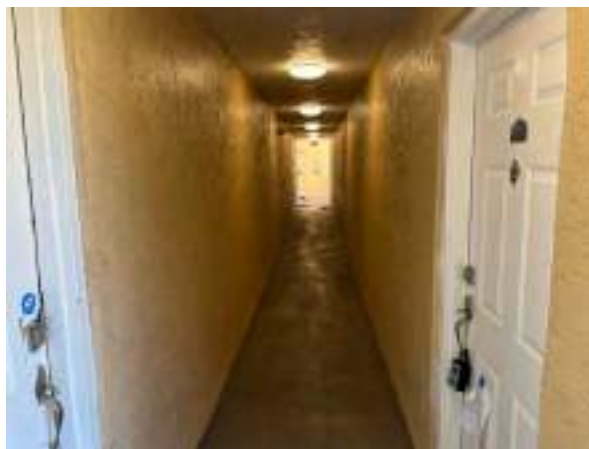
Typical view of covered open air corridor. Reserves provides for painting, waterproof membrane replacement, and replacement of lighting fixtures.
