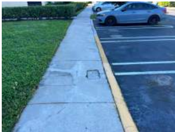
Community curbs, gutters and sidewalks are Association responsibility. Reserve provides for these components to be repaired as needed.
