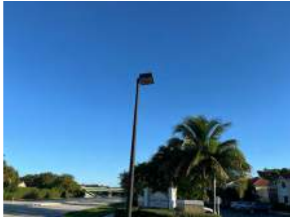
Entry for street lights considers poles, wiring, fixtures and controls will be repaired as needed. No assumption all units will need to be replaced at the same time.
