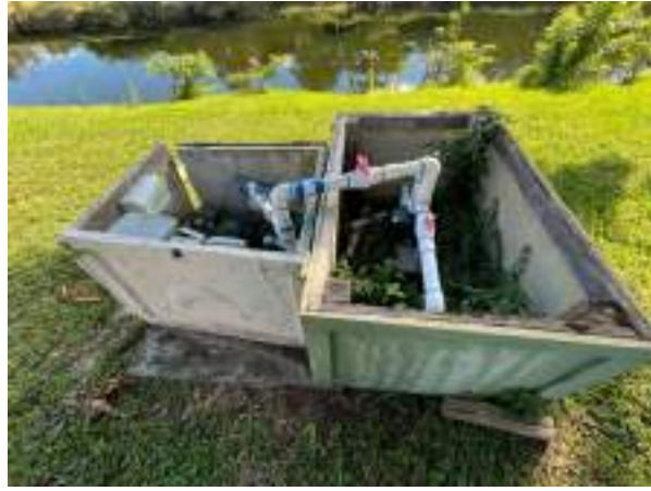
Irrigation systems can be kept in service by replacing failed sprinkler heads, piping, valves and controls, as needed.
