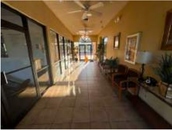
View of entrance/hallway of clubhouse. Repair/replacement components include flooring, ceiling fans, and light fixtures.
