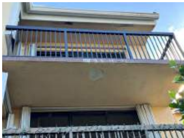
Concrete balcony repair cost can be expensive if failures go undetected and corrective action is not taken in a timely manner. See "Comments" section for additional information.
