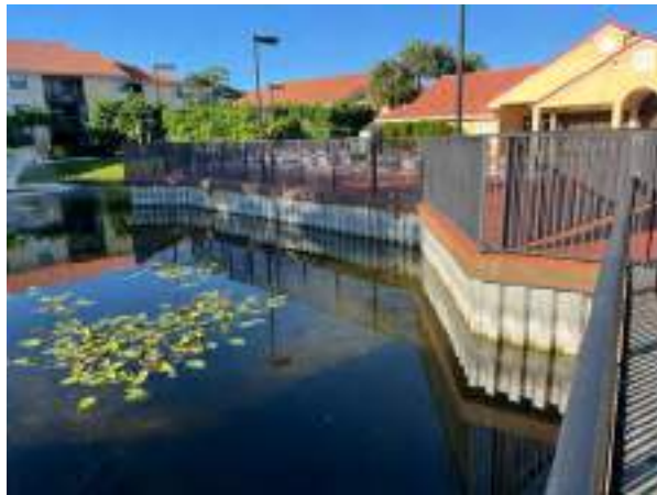
Retaining wall at pool deck will eventually require replacement. Reserves provides for this work when needed.
