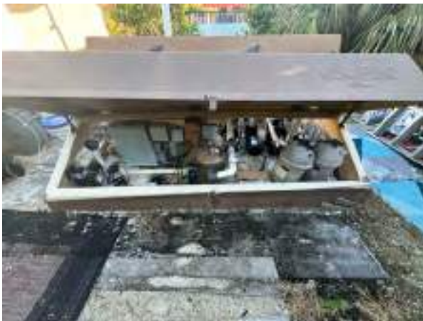
Reserve provides for repair/replacement of pool filters, water supply/return piping, chemical equipment and other system components.
