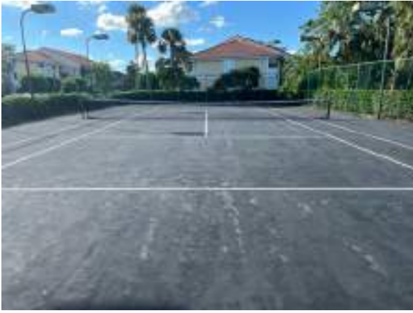
Tennis courts need periodic crack sealing and color coating. Major repairs are needed when cracks and surface areas deteriorate and detract from play.
