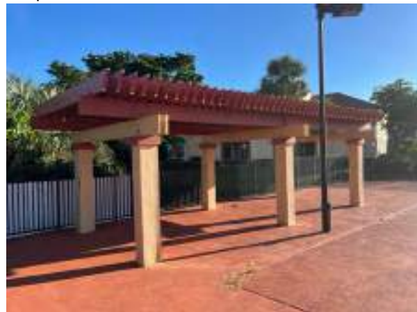
Trellis located on pool deck is in good condition. Reserve provides for repairs to masonry columns and replacement of wood trellis when needed.
