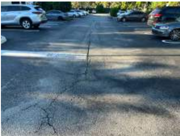
Asphalt pavement is nearing end of useful service life; association should plan on mill/overlay in near term. See our recommendations in comments section to maximize pavement useful life.
