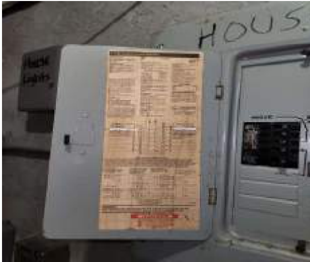
Branch circuits (panel electrical room)
