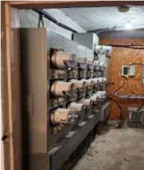
Electrical service equipment
