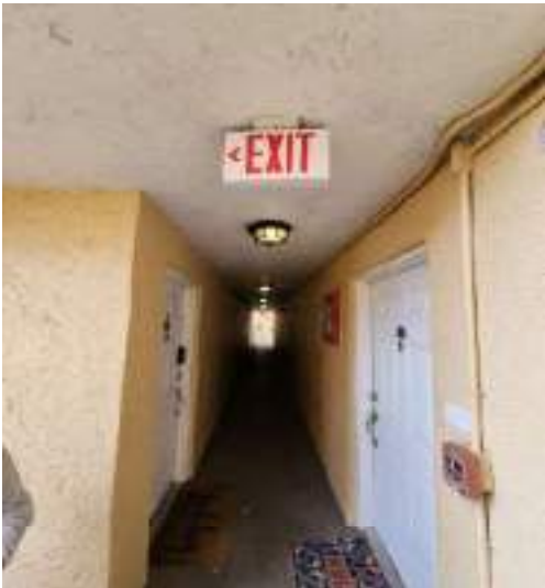
Building egress illumination
