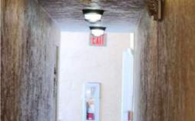
Building egress illumination
