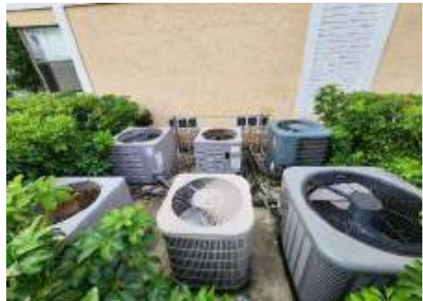
Mechanical equipment disconnect
