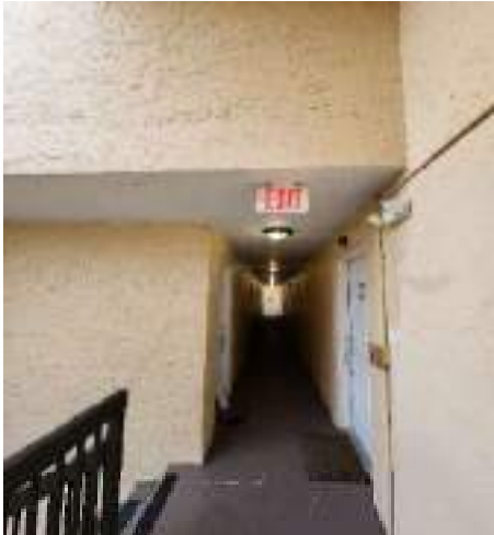
Building egress illumination
