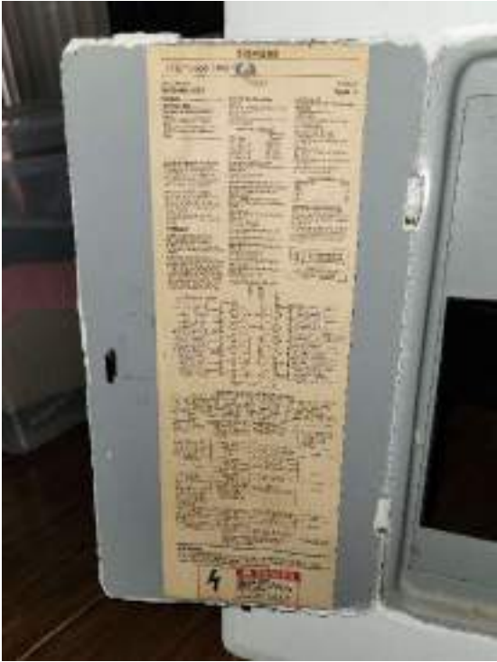
Electrical panel in unit 302
