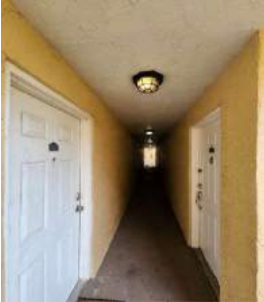
Building egress illumination
