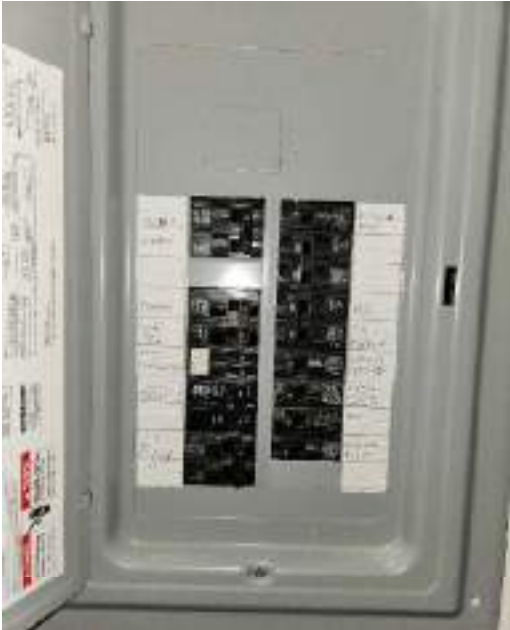
Electrical Panel (Unit 204)
