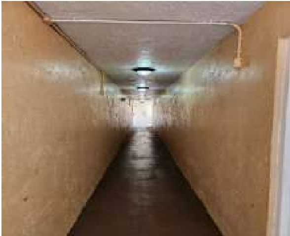
Building egress illumination
