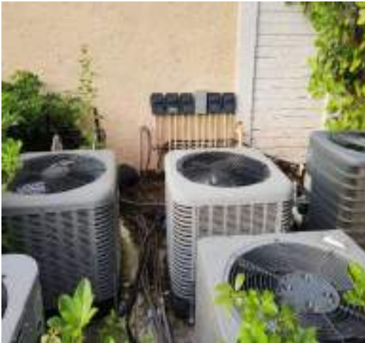
Mechanical equipment disconnects
