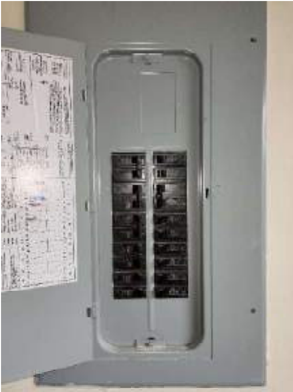
Electrical panel in unit 106
