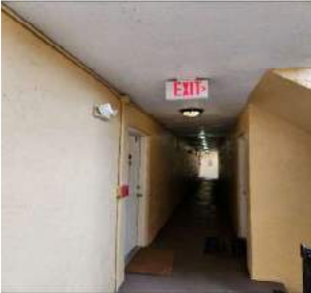
Building egress illumination
