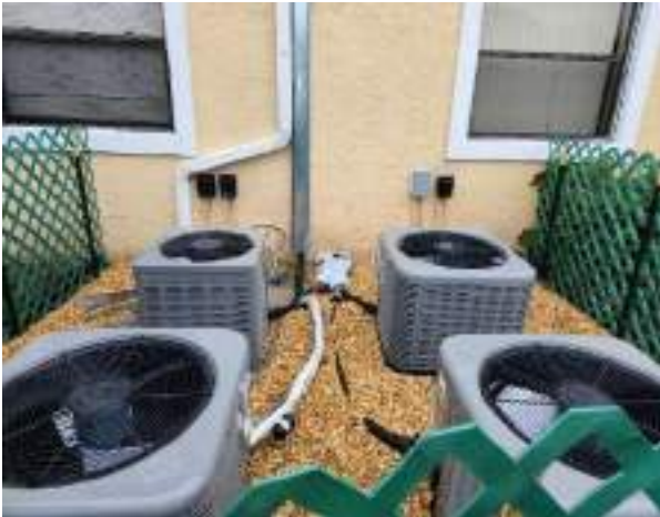
Mechanical equipment disconnects
