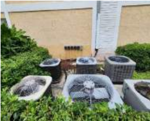
Mechanical equipment disconnect
