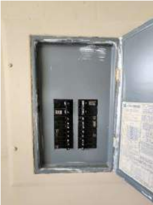
Electrical panel in unit 201
